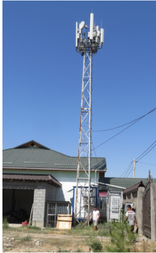
Fig.8 - Antenna-mast structure of the mobile operator
