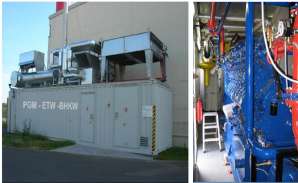
Figure 6 - Mobile methane utilization units PGM-ETW 1360 MG
