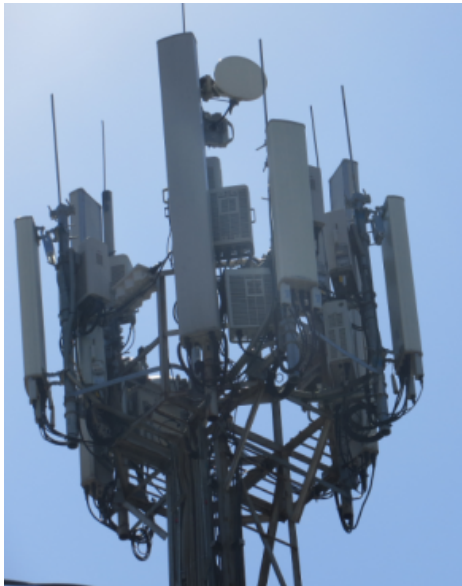
Fig. 11 - Placement of antennas on AMS
